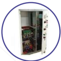
Solar Energy Power Cabinet
